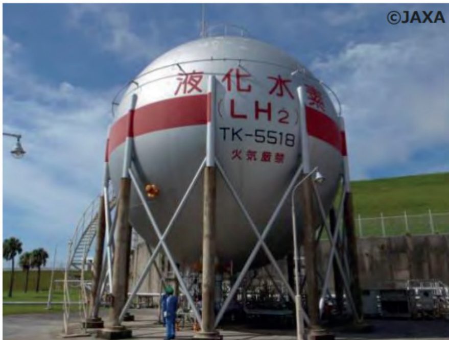
Figure 43: Spherical storage tank – Jaxa
